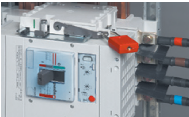
^ Draw-out DPX 630 immobilised using padlocks
