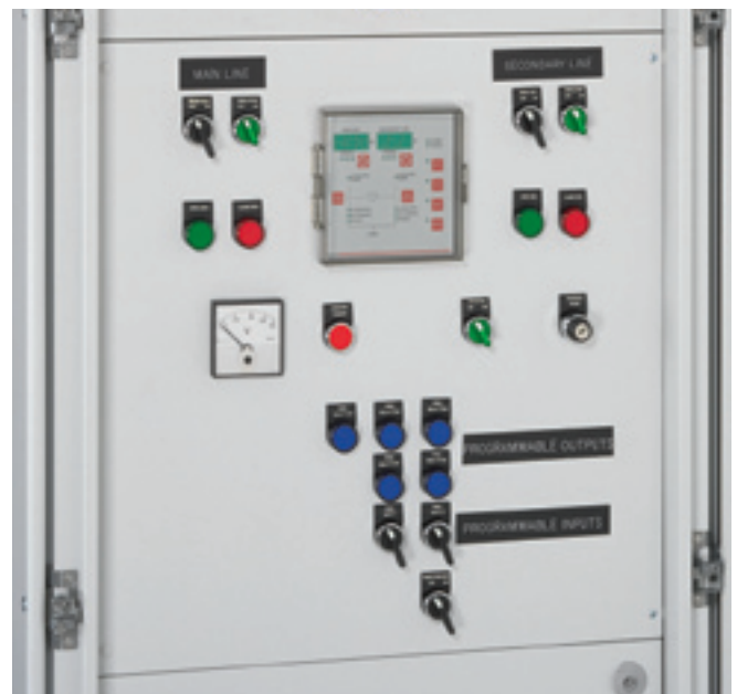
Supply inverter > control panel with control unit
