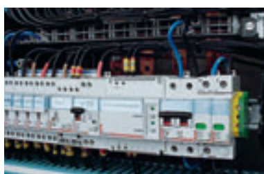
< Using a Lexic distribution block enables easy connection of a voltage surge protector for protecting a group of circuits
