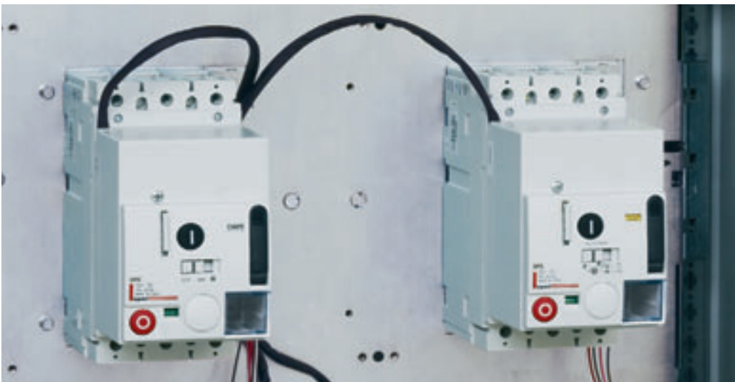
< DPX 250 mounted as supply invertors with motor-driven controls
